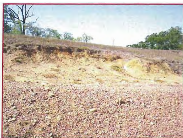
Photo 10 – Erosion scarring along the gully banks
