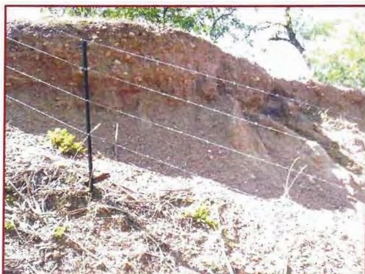
Photo 9 – Erosion scarring along the gully banks
